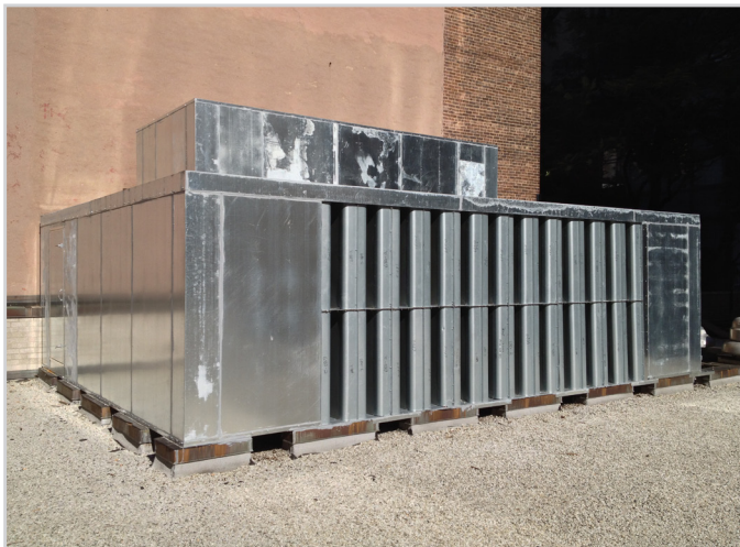
Custom Price Acoustic Enclosure at 1230 3rd Avenue New York, NY
